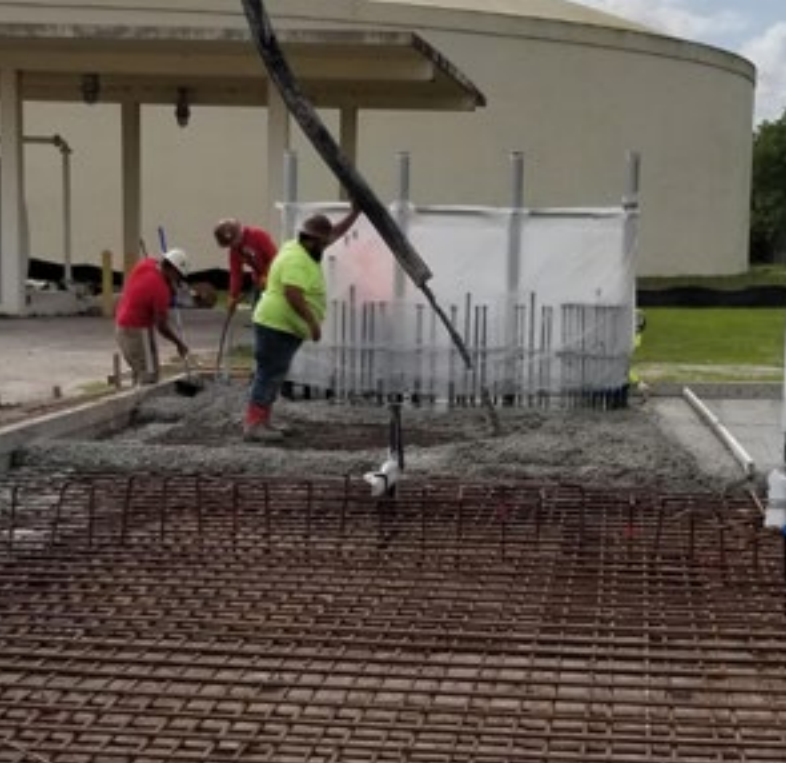
Foundation concrete pour for the degasifier scrubber project at the water production plant.
