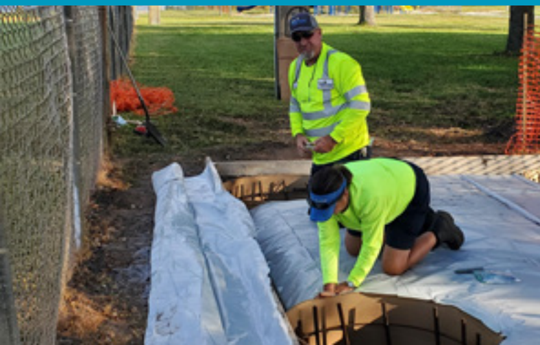
Employees Working on New Dugouts at Eddie Lee Taylor, Sr. Community Complex
